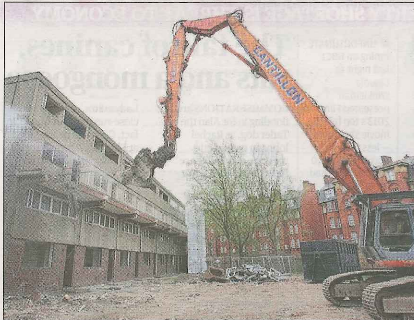
First blow: the bulldozers start work on Southwark's Heygate Estate in April 2011
